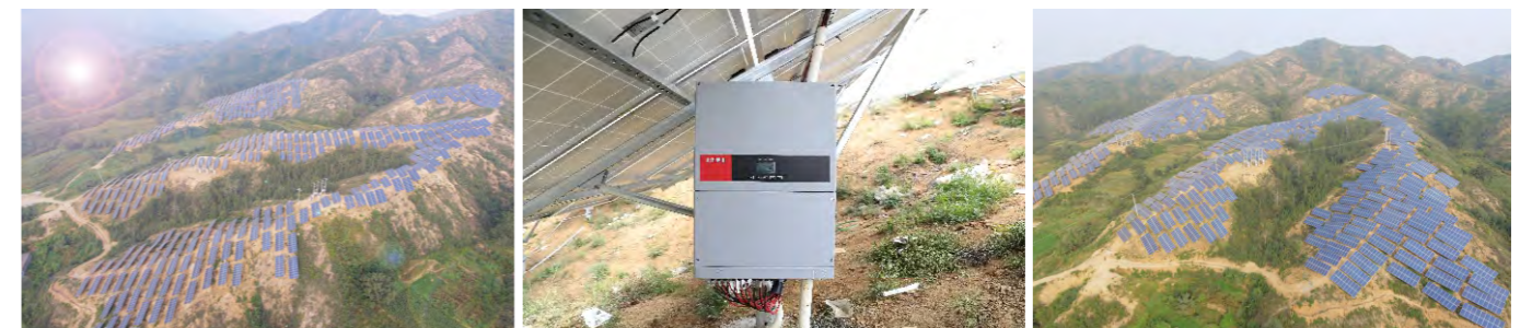
4.5MW p Inverters: 90* Suntrio Plus 50K Address: Shijiazhuang Hebei
