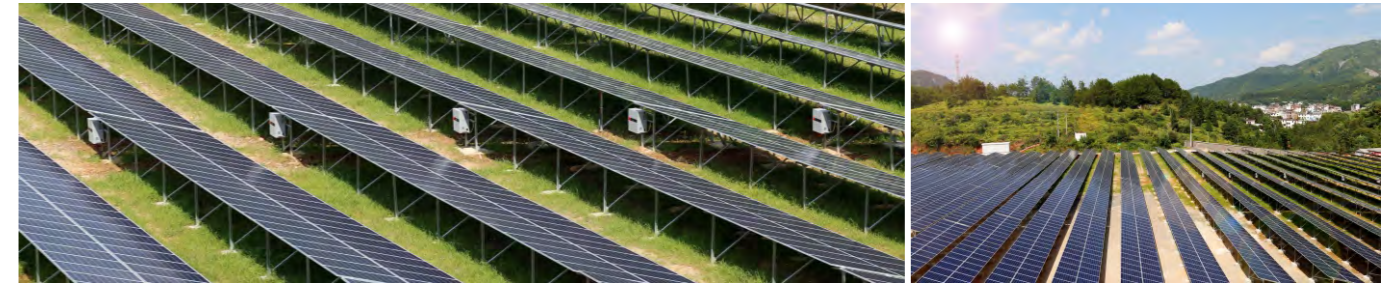
1.6MW p Inverters: 27* Suntrio Plus 50K Address: Shangyou Jiangxi
